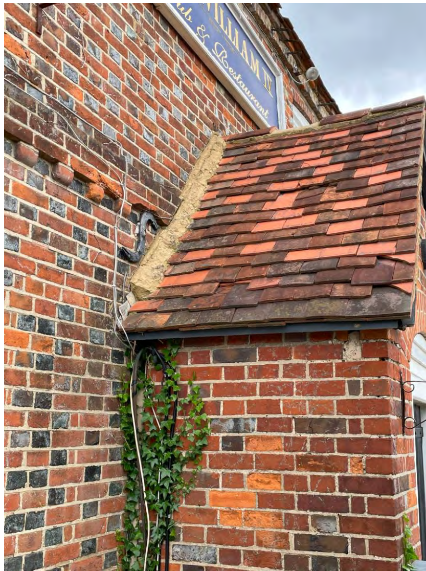
Figure 20: Porch brickwork is clearly different from that of the original building.
